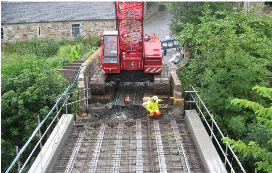
The overall length of the deck is some 9.5m, with a clear span of 7.6m and overall width of 5.85m.
